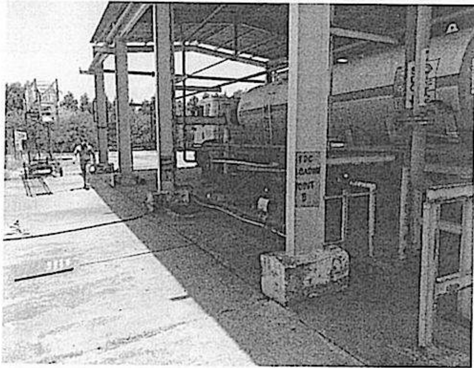
EDC Loading tanker driver observes swivel joint upstream side leak 1.1
