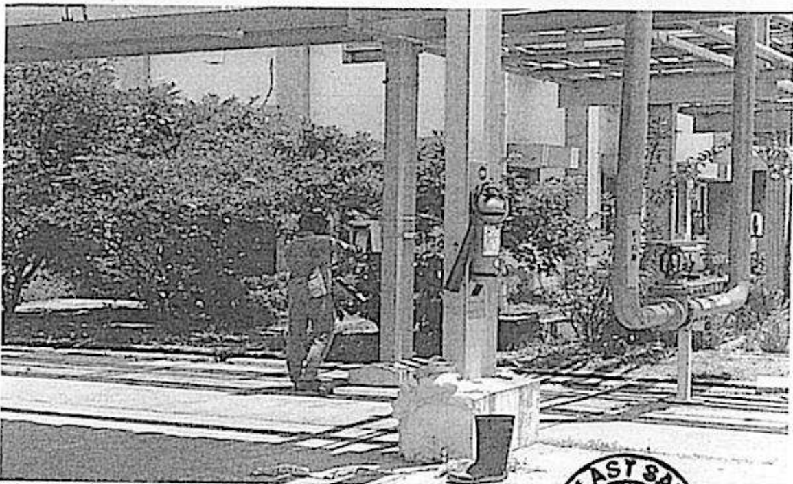
Driver presses the emergency button to shut down the loading pump operation and informs the area officer 1.2
